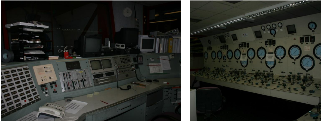
Figure 2.3/2.4: Two pictures of the Saturation Diving Chamber Control Centre at the National Hyperbaric Centre in Aberdeen. The right picture shows the controls relating to the delivery of the breathing gases to the chamber. In the left picture the control for interaction with the divers is shown (the chamber can just be seen through the glass). Both Pictures Copyright Hugh Finlayson (2008).
